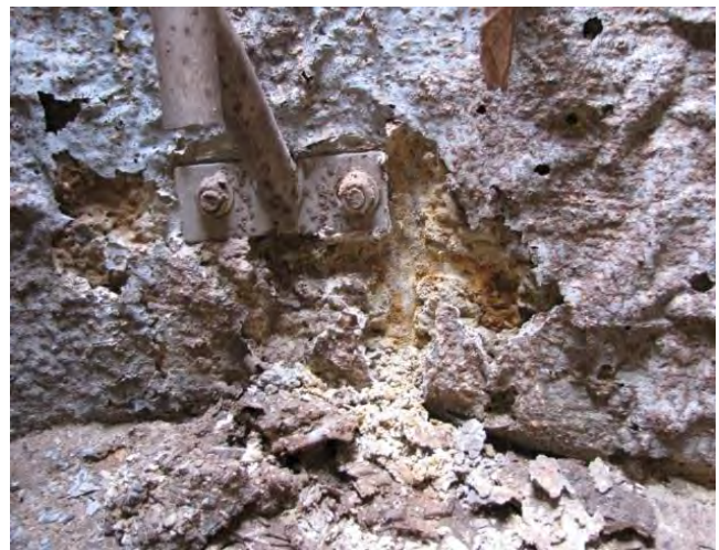
Figure 5 Corrosion around ladder
