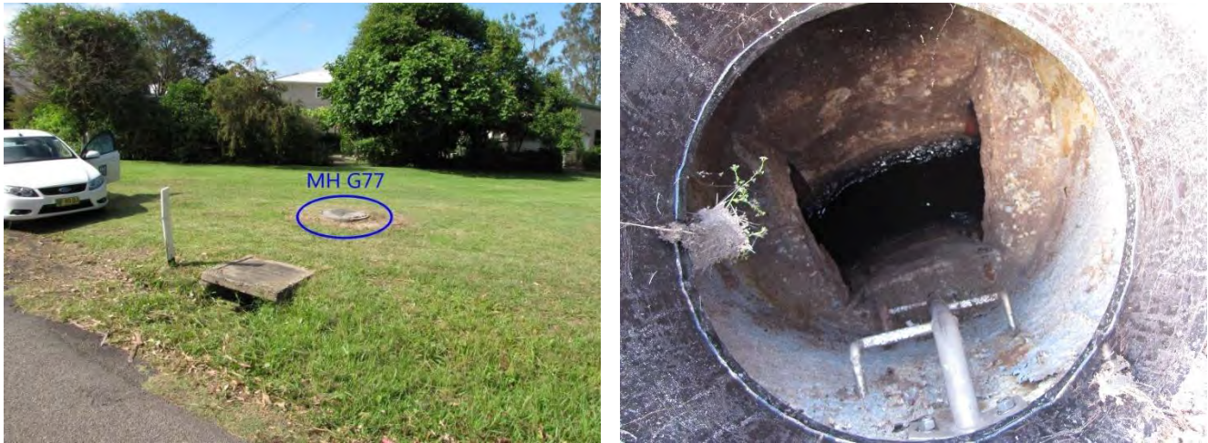
Figure 3 showing blistered/ missing coating and corroded concrete– 29/10/15
