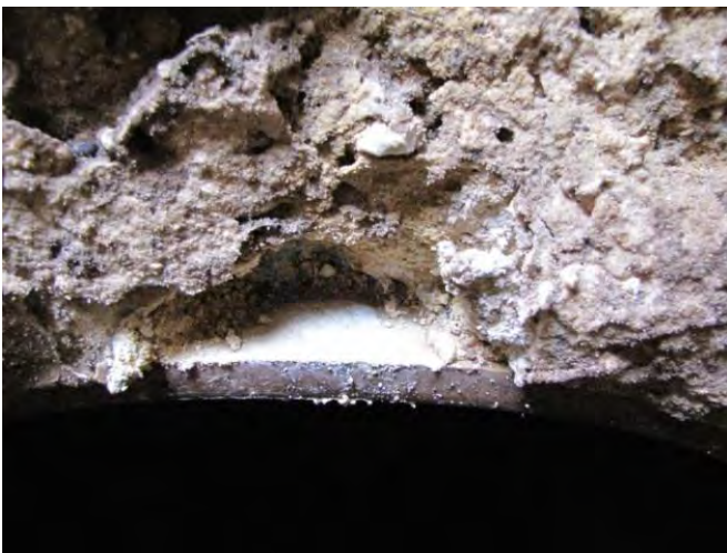
Figure 4 Corrosion above GRP pipe
