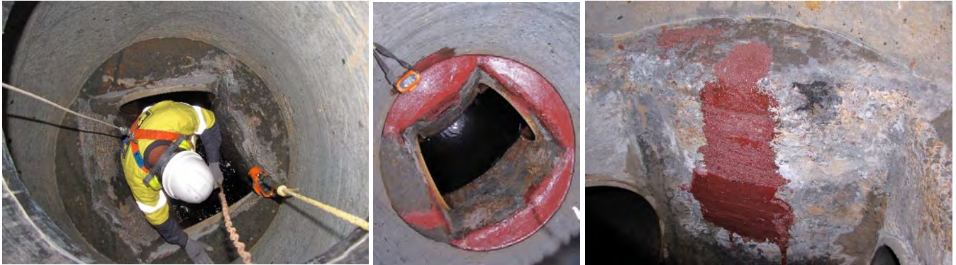
Figures 6, 7, 8 - After high pressure water blasting, corrosion damaged benching was rebuilt using Metz 10EN
