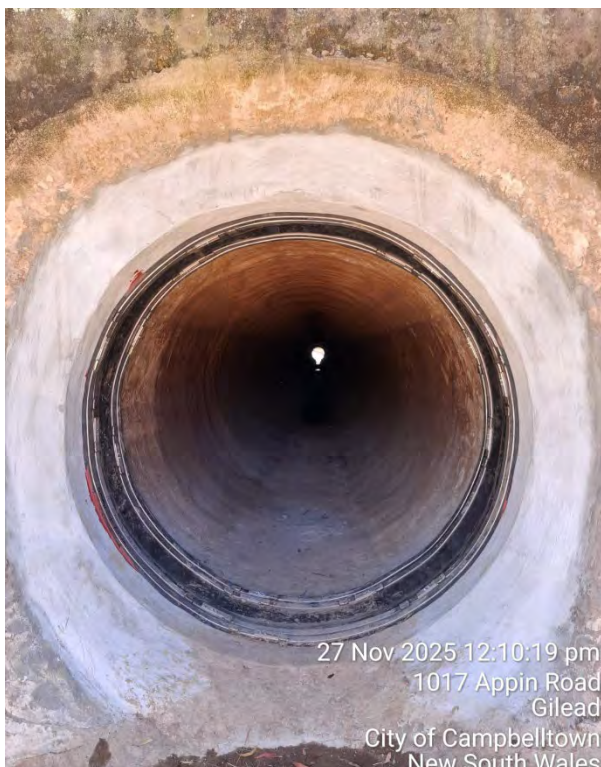
27 Nov 2025 12:10:19 pm 1017 Appin Road Gilead City of Campbelltown New South Wales Figure 6 HydraTite Seal installation complete Nov 2025 Photo Courtesy of Interflow
