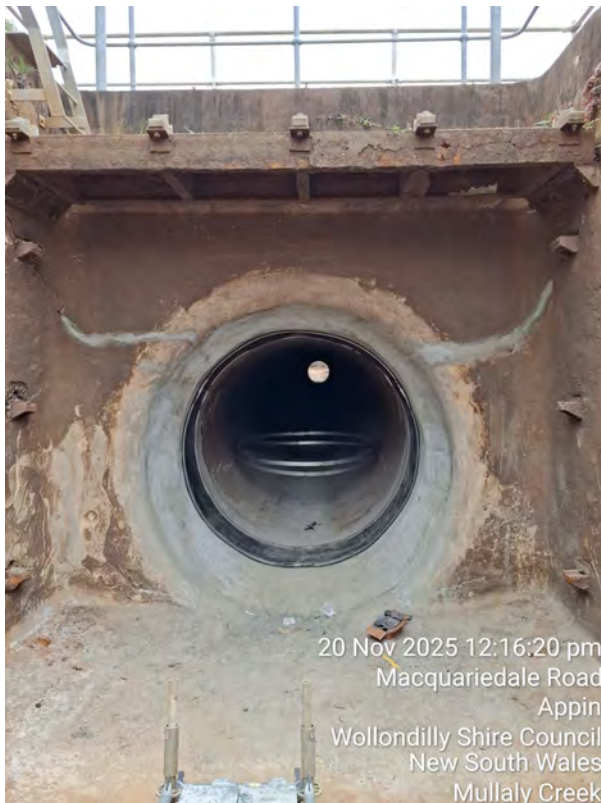
20 Nov 2025 12:16:20 pm Macquariedale Road Appin Wollondilly Shire Council New South Wales Mullaly Creek Figure 4 HydraTite Joint Seal partially installed, Nov 2025 Photo Courtesy of Interflow
