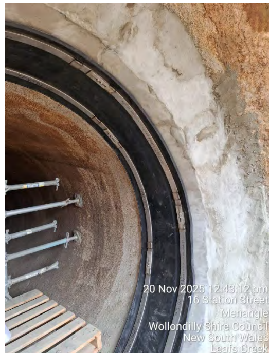
20 Nov 2025 12:43:12 pm 16 Station Street Menangle Wollondilly Shire Council New South Wales Leafs Creek Figure 5 Closeup of HydraTite Seal partially installed Nov 2025 Photo Courtesy of Interflow
