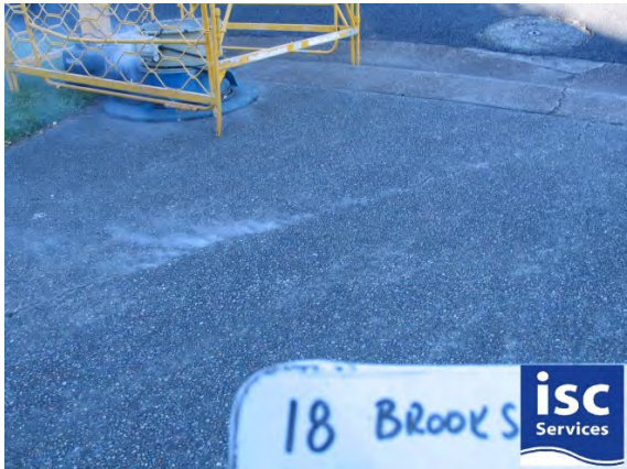
Figure 12 Smoke from cracks in a driveway – I/I source
