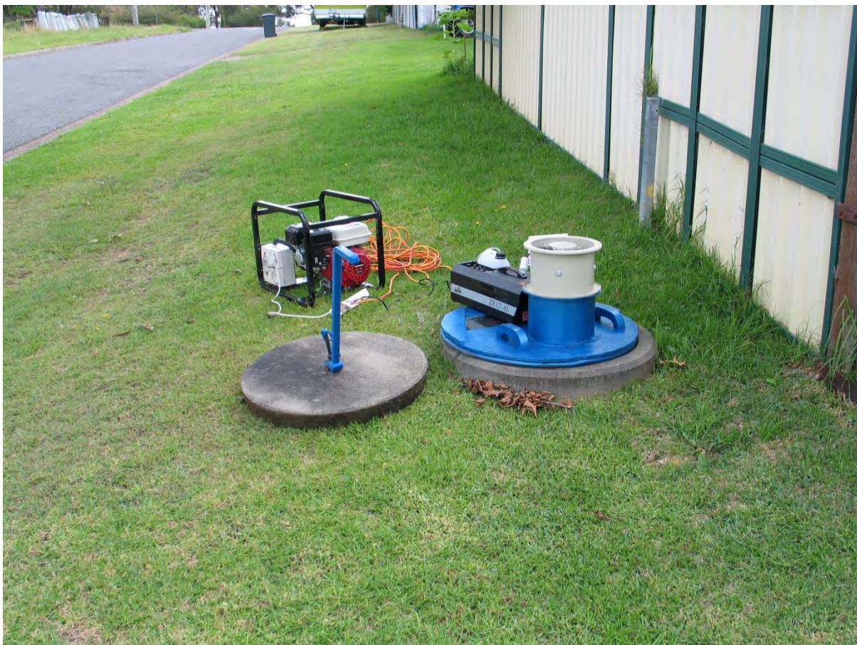
Figure 6 Smoke generator and fan arrangement – positioned ready to introduce smoke into sewer
