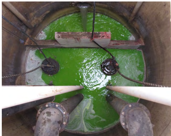
Figure 17 Green dye flowing into pump station
