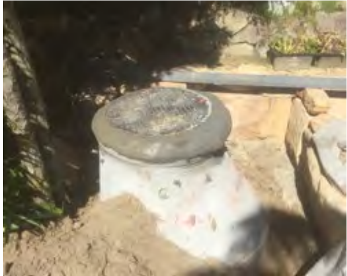
Figure 2 mortar around new cast iron frame
