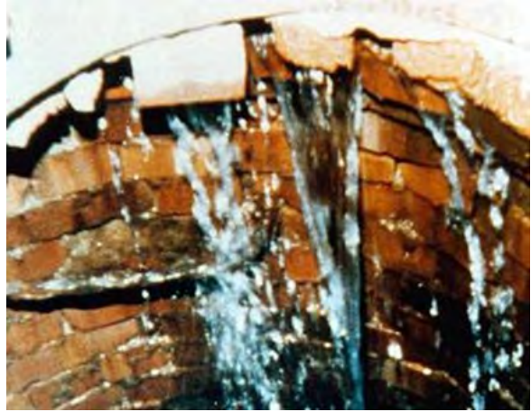
Figure 15 Blue dyed water infiltrating through damaged brick riser section
