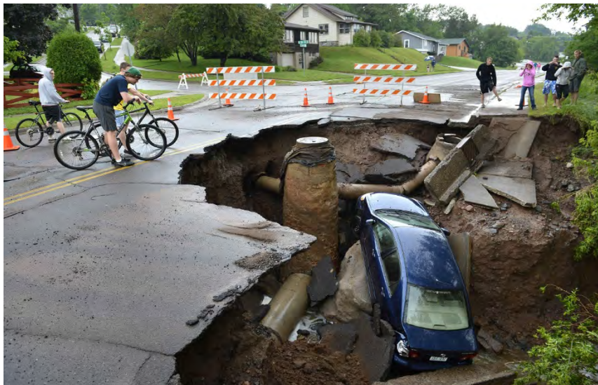
Figure 3 Extreme example of what can happen with soil movement over time due to infiltration and exfiltration leaks in sewers and stormwater systems
