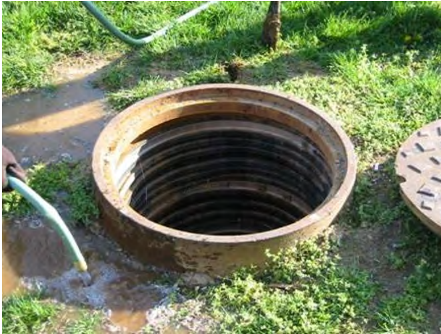
Figure 18 Ground around the MH is saturated and joints observed for seal
