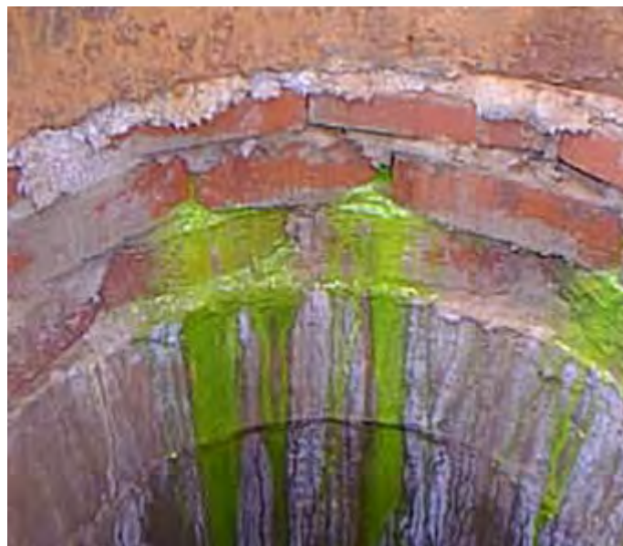
Figure 13 Green dye infiltrating through damaged mortar of a brick riser section
