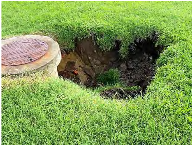
Figure 4 showing a serious large void due to infiltration leak. Image and report posted by ssellen, 10 January 2017, Daily Mercury
