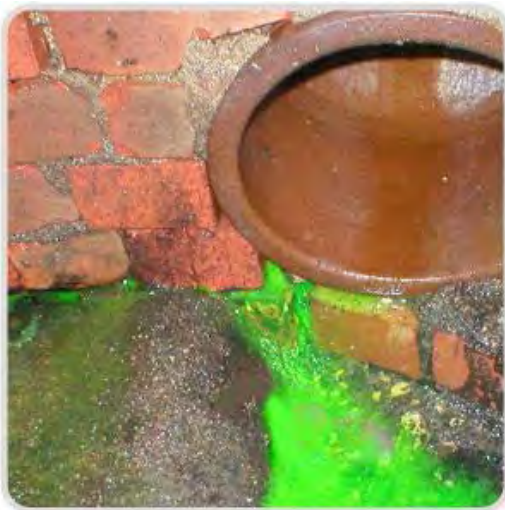
Figure 16 Green dye infiltrating from the wall penetration
