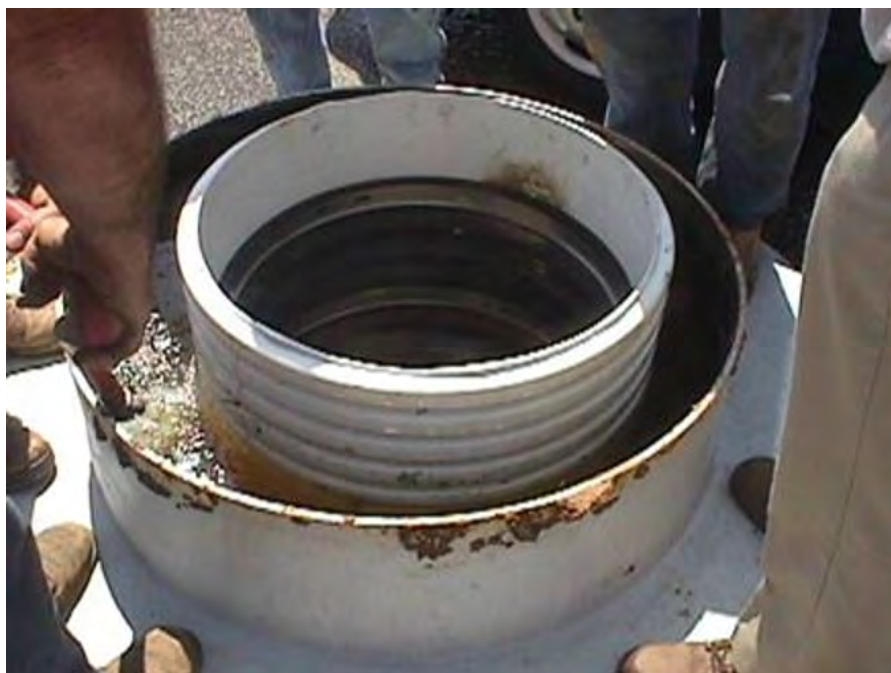
Figure 19 Water is introduced into the space around the MH on a hard stand and observation made to determine quality of joints seals
