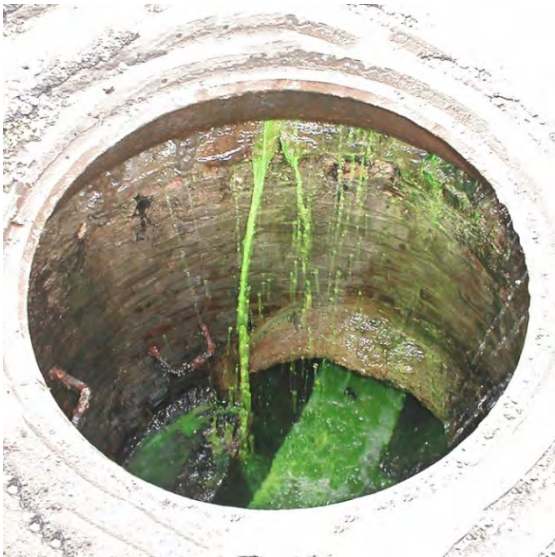
Figure 14 Dyed water flowing in through the frame and shaft
