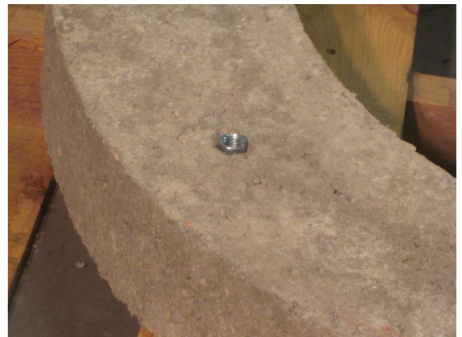
6. If using drop in internally threaded anchors, place the anchors in each of the previously drilled holes.
