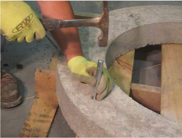
7. Lock in the drop in internal threaded anchors using the drop in anchor setting tool and a hammer.
